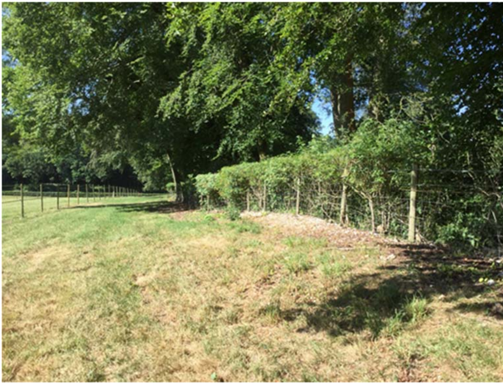
Photograph 7.14.11. A boundary feature intersected by the Order Limits, bordered by grazing fields. (Site 5, north, 27/06/18, standard lens).
